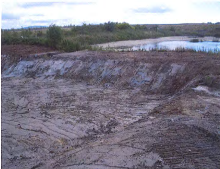
Inlet lagoon cleaning in in the foreground while the main lagoon is fully operational in the background.
